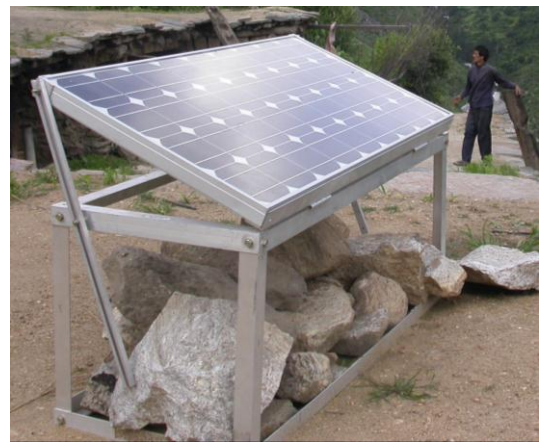
Figure 6 Solar panels with manually adjustable tilt angle.
