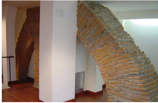
Figure 6 Lighting of the old chimneys, attic of Black Eagle building
